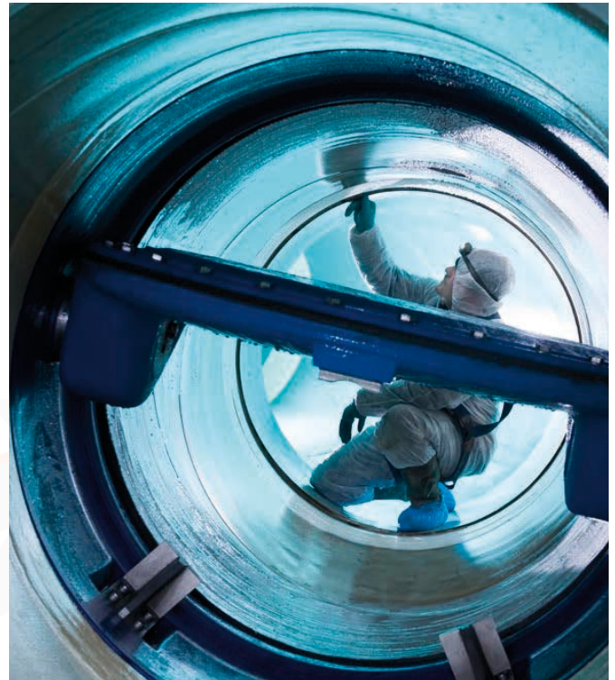
The West-East Link Main is a new pipeline between Liverpool and Manchester that United Utilities built a few years ago to provide better connectivity and enable them to operate the water network in a more integrated way, allowing flows to be diverted when needed
